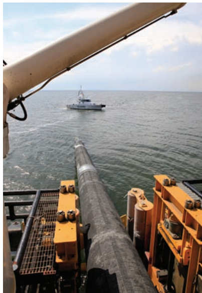
Saipem's Castoro Dieci pipelay vessel worked in the Bay of Greifswald, Germany, from June to October 2010. Designed to operate in shallow waters, it installed 28 km (17 mi) of each of the twin pipelines in that area. Photo courtesy Nord Stream.
